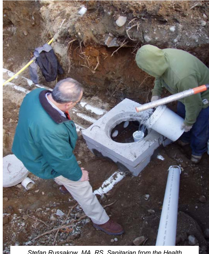
Stefan Russakow, MA, RS, Sanitarian from the Health Department checks a distribution box for a new septic system
